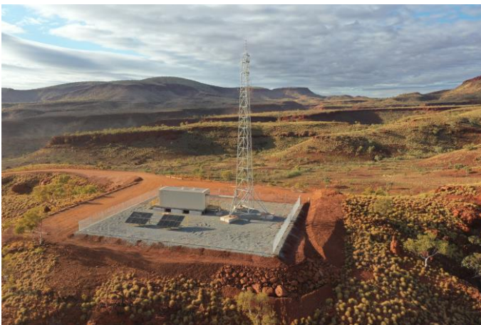
A Radlink telecommunications tower
